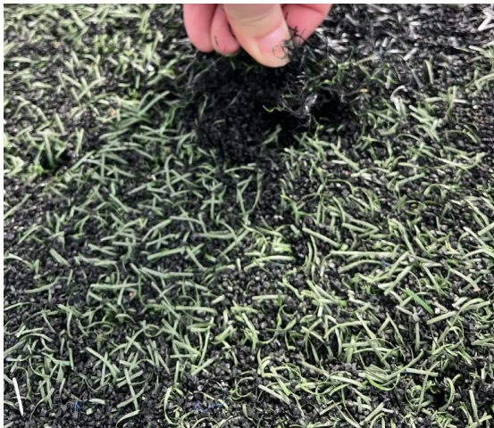
The 2026 photos to the left and below illustrate many tears that have developed over the past five years. While photos can't quite show the full extent of the damage, the tear in the photo to the left extends toward the lower right and left center of the picture, creating a "flap" that is disruptive to lay and potentially dangerous to athletes.
