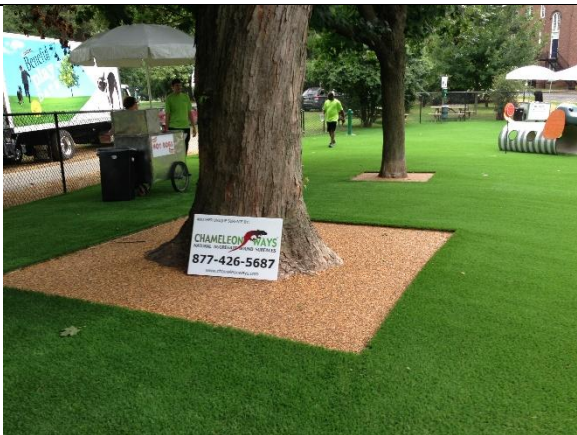
City of Lancaster, PA Addapave tree pit material to fix the aggregate in place and still maintain porosity for healthy tree growth.
