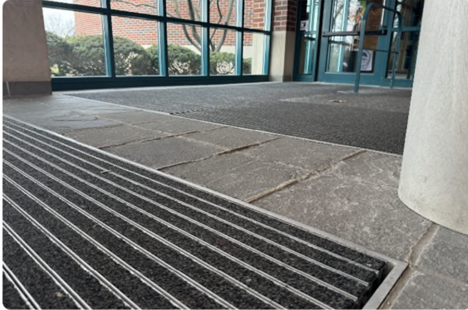
The library building is over 30 years old and needs crucial repairs and updates to meet ADA compliance and modernization.
